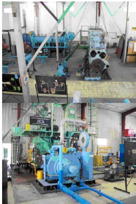
Internal combustion engine workshop
