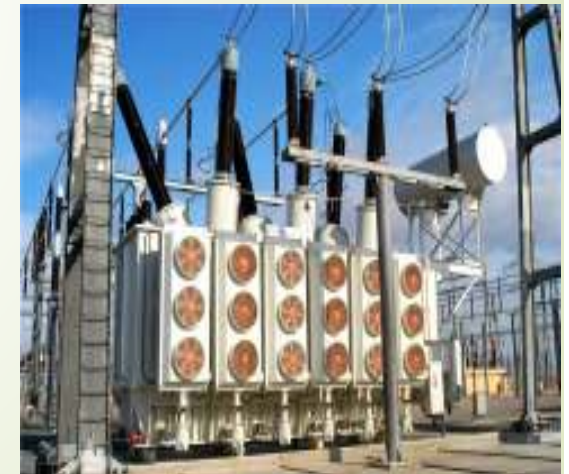
Substation power transformer
