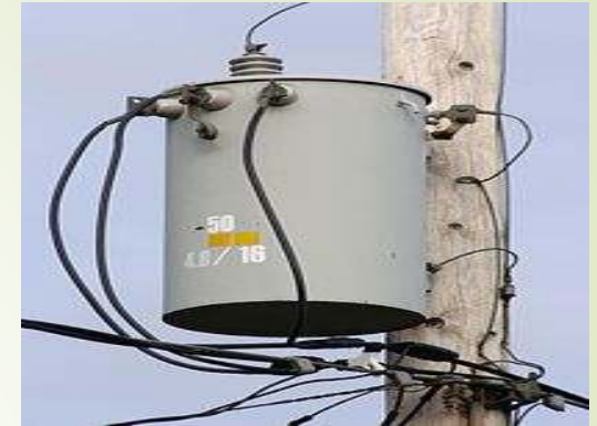
Pole mounted single phase distribution transformer
